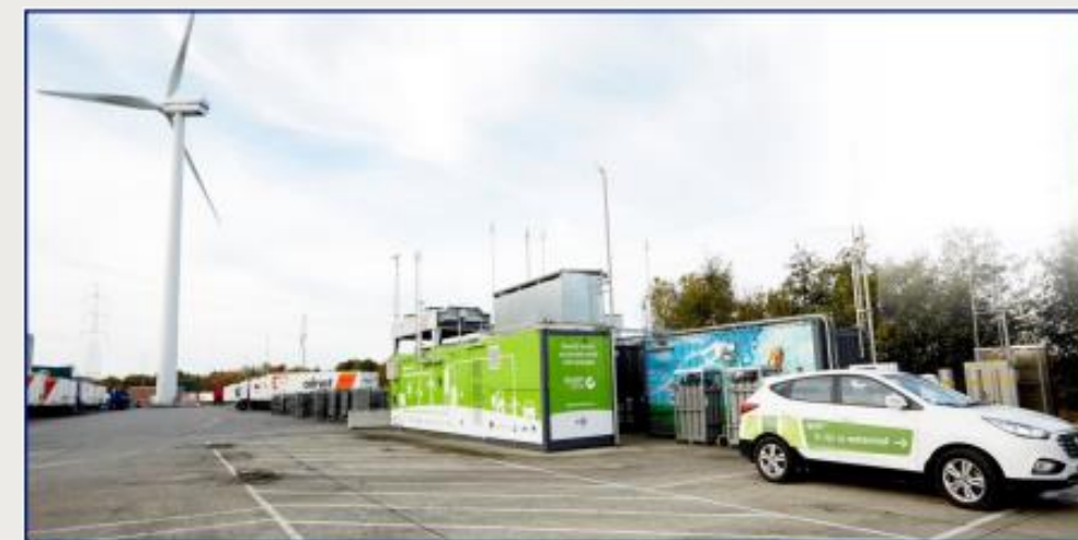
Colruyt Group, Halle (Electrolysis +RE)
